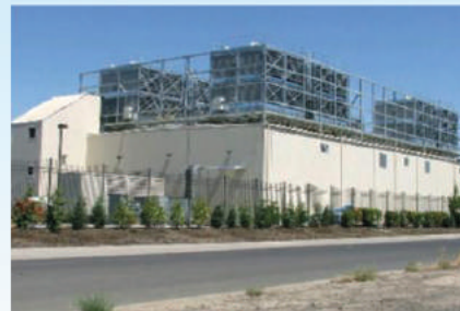
Google data center = Warehouse-scale computer
